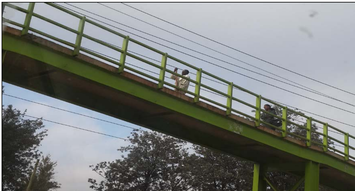
Plate 5.5: A PWD using a section of the Foot Over Bridge to cross the Thika Superhighway.
