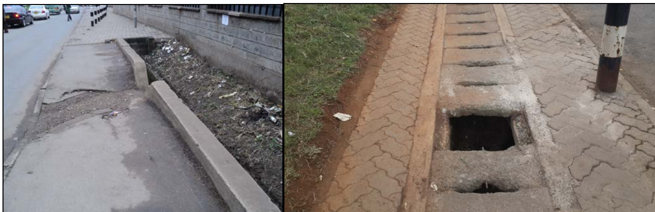
Plate 5.1: Sections of the poorly designed and maintained footpaths in Nairobi City
